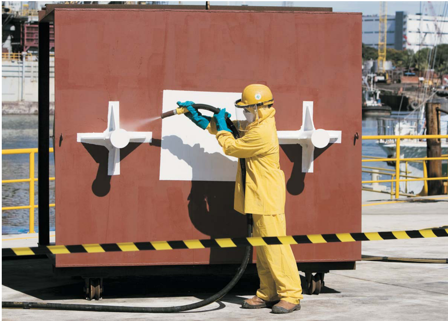
New technology: Using the Quill Falcon D-WAB system for wet blasting. A compressed air-propelled abrasive and water mixture prepares ship's surfaces
